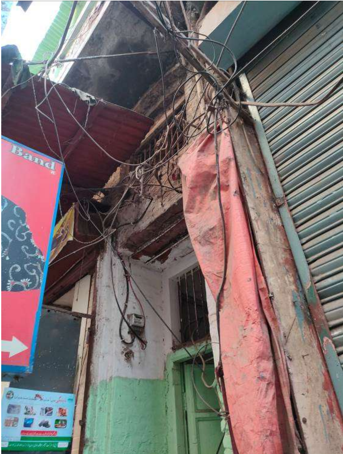
Tangled web of wires mounted onto the façade in a haphazard manner.
