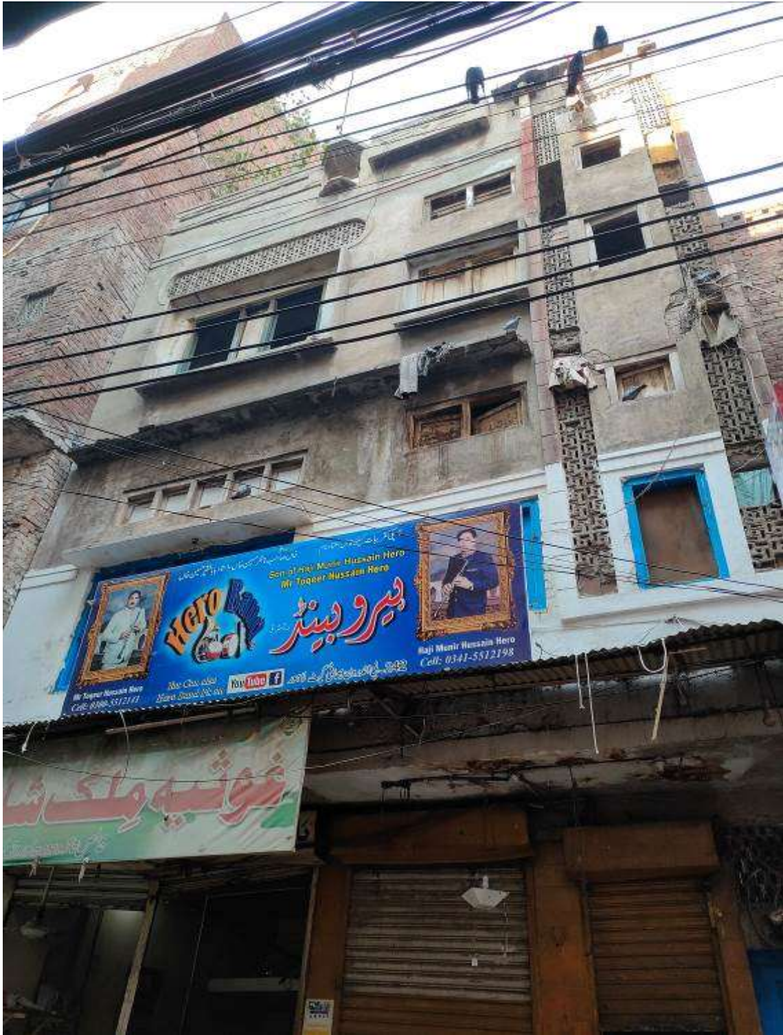
Some buildings still retain the original character of the historic fabric, but are in a state of disrepair.
