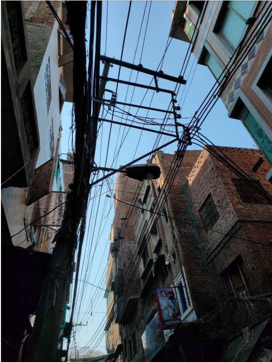
Electrical cables mounted onto posts and distributed overhead into different streets.
