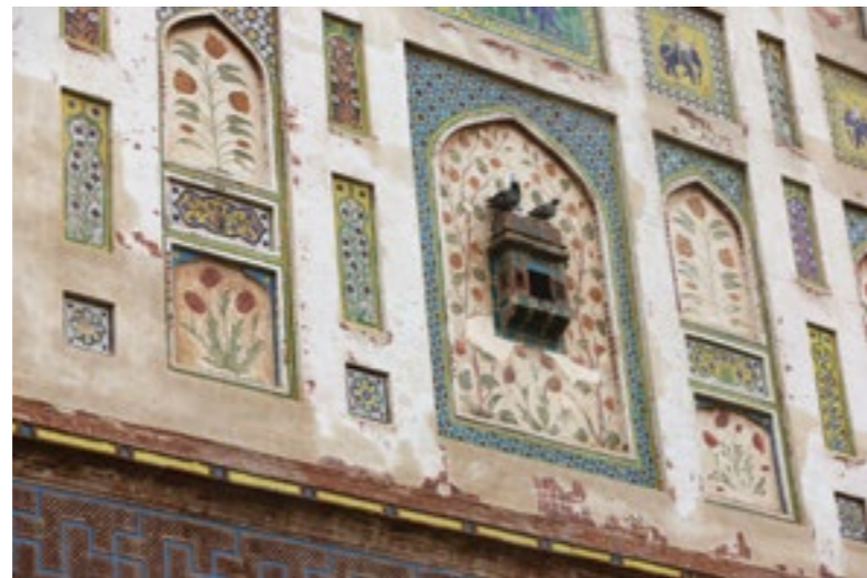
Close up of decorative features of restored western section of Picture Wall
