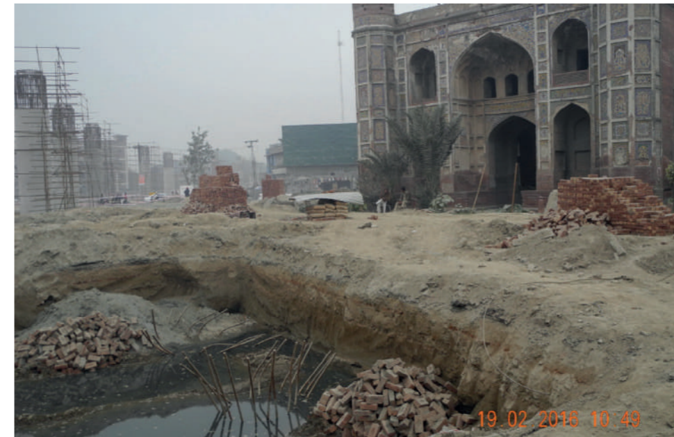
Pit cut for one of the Orange Line's viaduct piers in front of Chauburji. Image: Maryam Hussain, 2016
