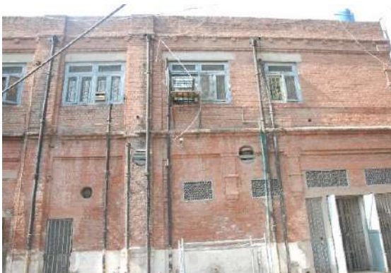
Figure 17 Deterioration of Structure
